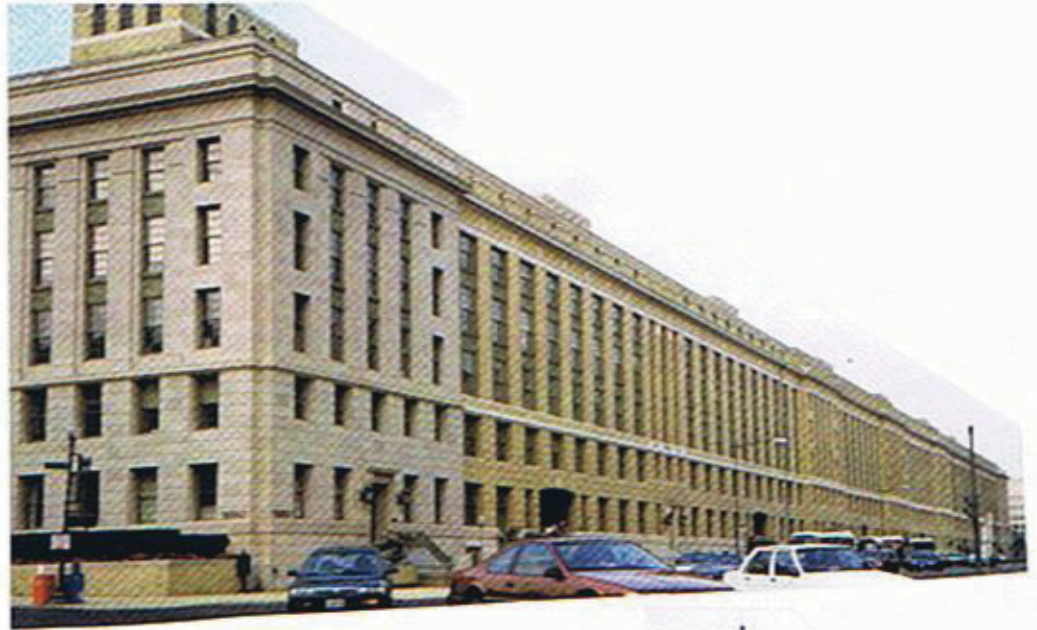
U.S. DEPARTMENT OF AGRICULTURE, SOUTH FACADE LOCATION: 13TH AND G ST. WASHINGTON DC DATE: MARCH 85 - NOV. 85 CONTRACTOR: Schlegel Corp., New York SCOPE: Restore 1,100 window frames and replicate sash.
